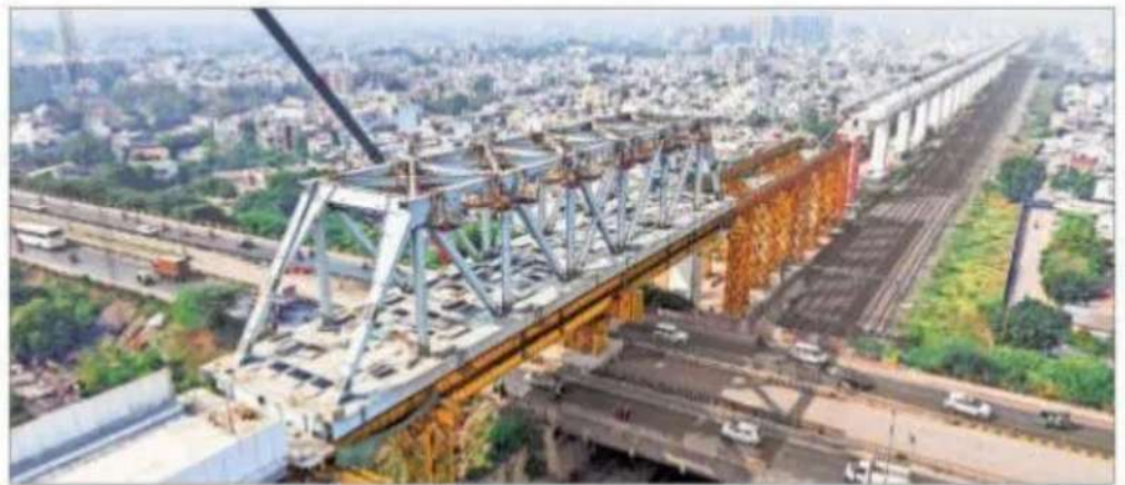
The 11th steel bridge has been launched over Cadilla flyover in Ahmedabad. EXPRESS
